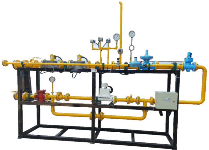
Low Pressure Pressure Reducing system with safety solenoid Valves along with Gas meter & Bypass Systems for automatic burners
